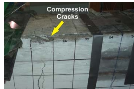
Fig. 10 Typical Failure on Concrete Compression
